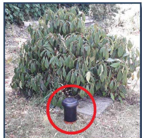
Poly-air installed on a septic tank ventilation pipe.
